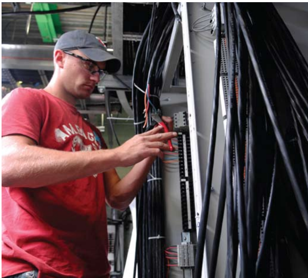
Jason Bjerke, apprentice technical maintenance technician, works on wiring a new protection upgrade panel during Young 2's electrical overhaul.
